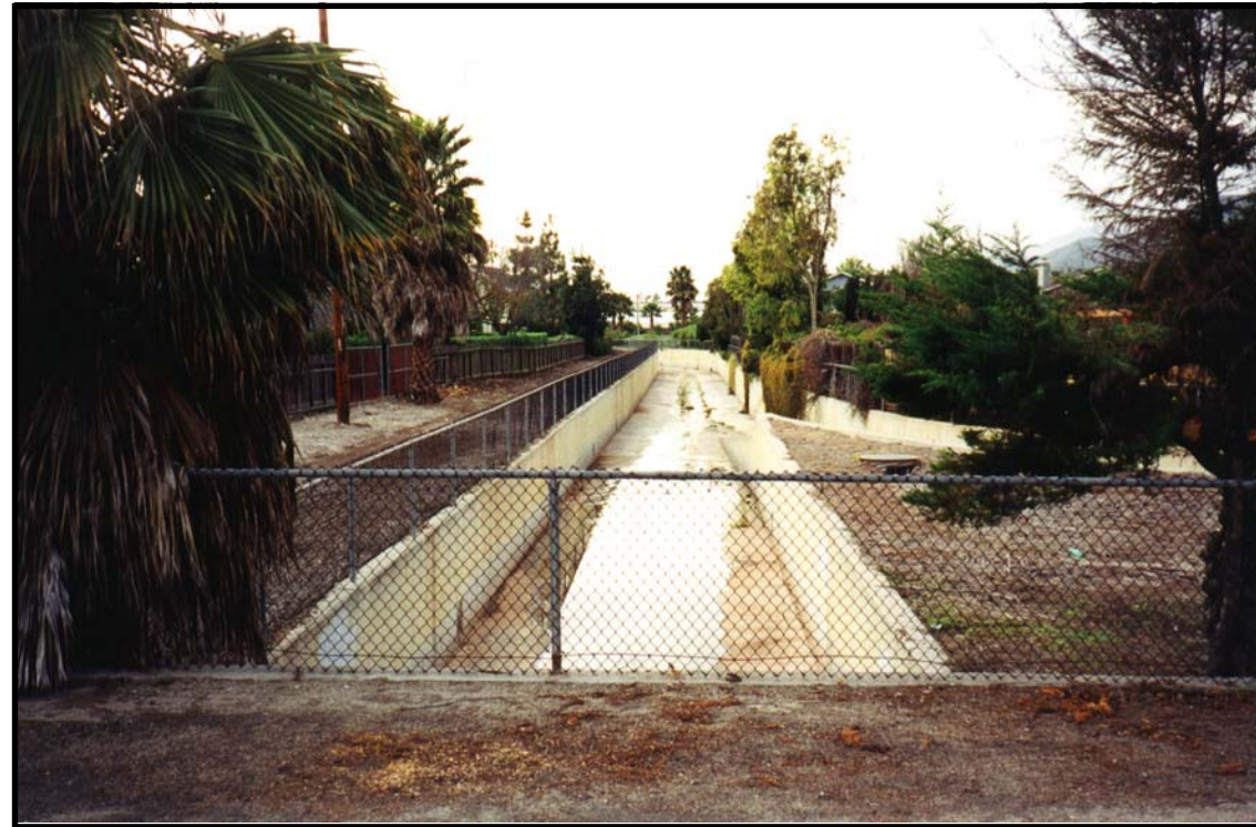
Looking west along the Main Channel of Franklin Creek, from near the Foothill Rd. / Linden Ave. intersection. The West Branch of Franklin Creek enters the Main Channel in the mid-ground of the photograph. These formerly natural creeks have been converted to concrete box channels.
